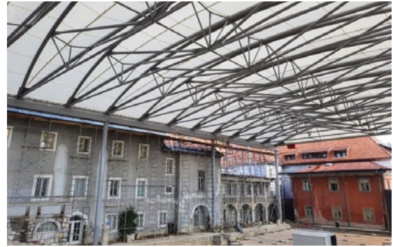
Gradnja nove strehe po načrtih prof. Petra Gabrijelčiča Construction of the new roof designed by Prof. Peter Gabrijelčič
